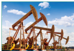
Oilfield Pumping Units
