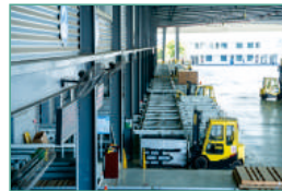
Logistics Conveyor System
